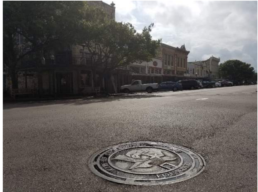
Stormwater system in the Most Beautiful Town Square in Texas
